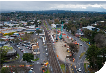
Aerial view of works to remove a level crossing and build a new transport hub in Croydon.
