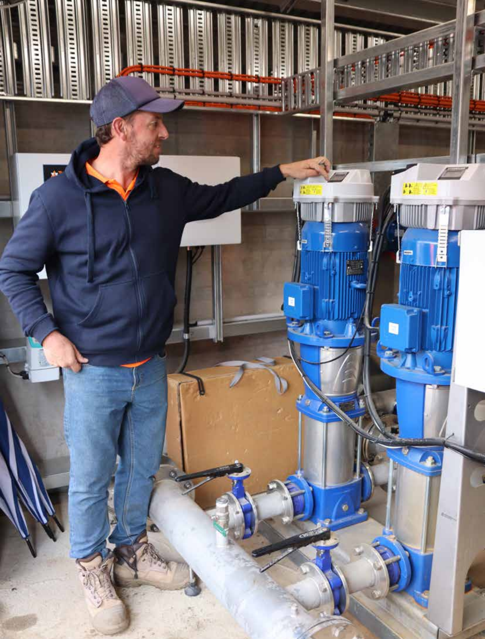
Storm water harvesting system in Croydon.
