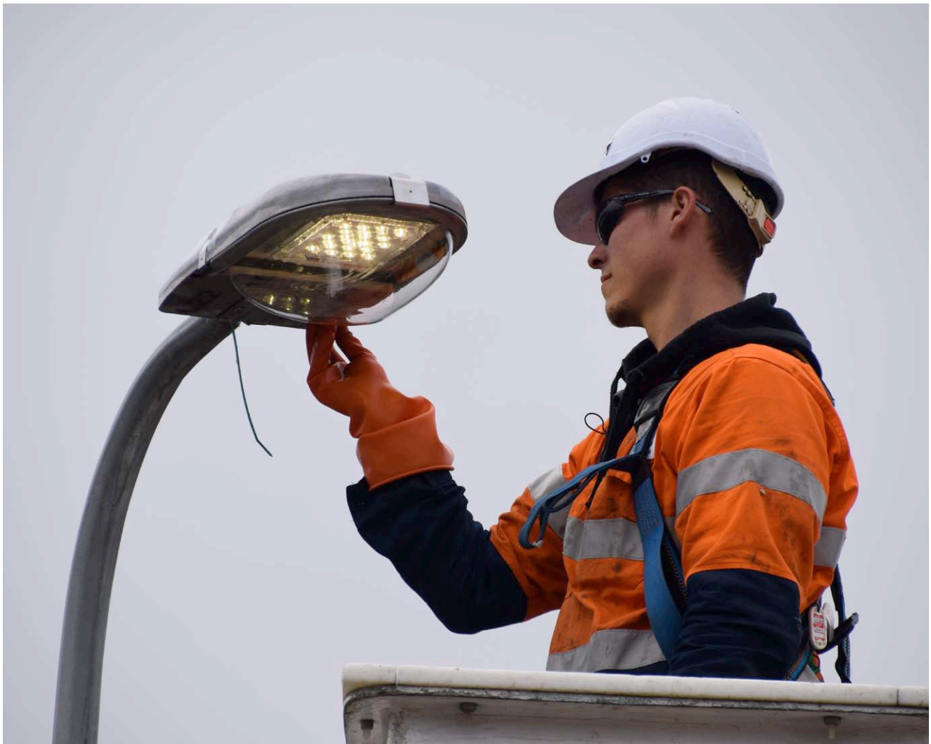
New LED street lights save 77 per cent more energy than the previous mercury vapour lights.
