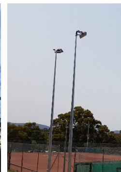
High mast LED Ringwood Central TC
