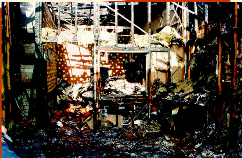
Fire damage at the Radio Station
